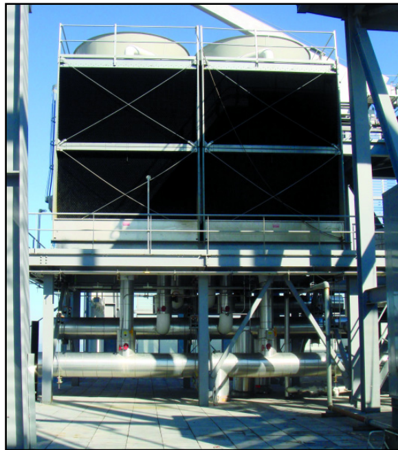
▲ A cooling tower atop a Manhattan office building is just one piece of the power and utilities equation being monitored by ERS's technology.
